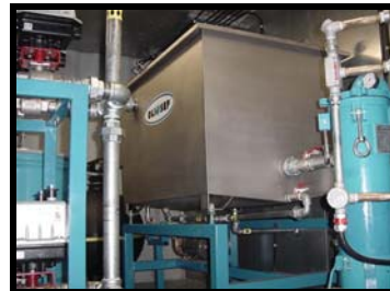
Filtration Separation Process
