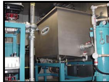
Filtration & Separation Process
